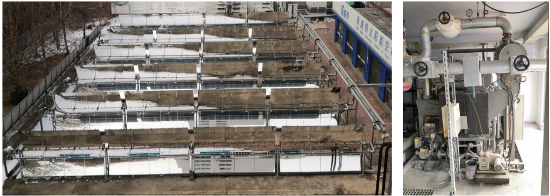
图 3 槽式太阳能集热系统和溴化锂吸收式制冷机组 Fig.3 Trough solar collector system and LiBr absorption refrigeration unit
